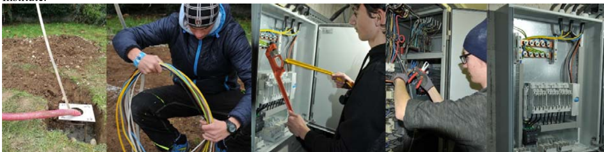
Picture 2: Preparation for setting up and connection of the charging station to power grid (Photo: S. Simović)
