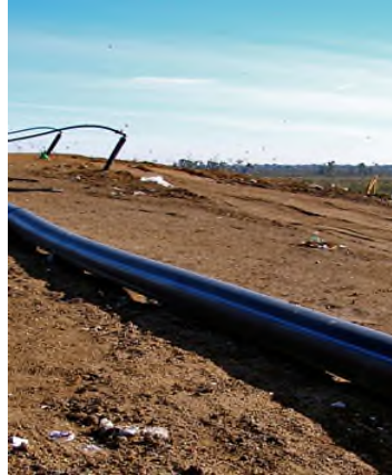
Figure 4: Pipes for gas collection and transport
