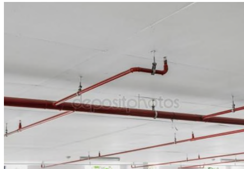
Figure 5. Dry sprinkler installation
